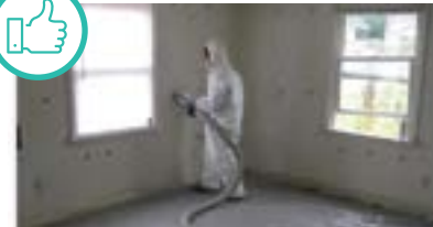
Insulating brick or stucco wall from interior. Courtesy of South Seattle College
