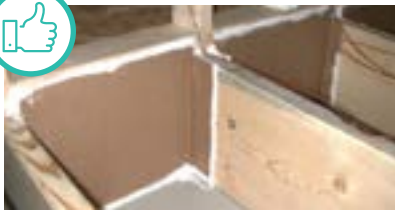
Floor joists under kneewall (blocked with rigid material and sealed with caulk). Courtesy of U.S. Department of Energy
