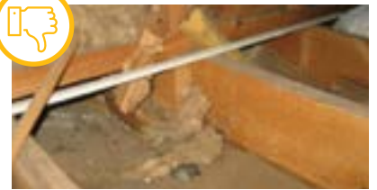
Floor joists under kneewall (not blocked with rigid material and unsealed). Courtesy of U.S. Department of Energy
