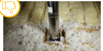
Unsealed penetration (heat-producing). Courtesy of U.S. Department of Energy Weatherization Program Trainers' Consortium (DOE WAP TC)
