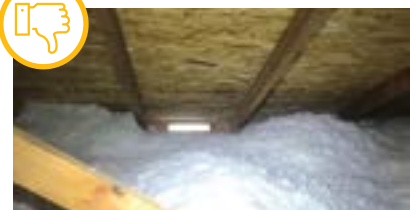
Roof-to-wall heel uninsulated. Courtesy of Advanced Energy
