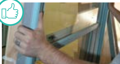
Proper fit window, level, and sealed. Courtesy of Santa Fe Community College
