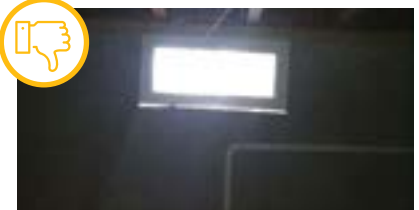
Window install not sealed, improperly fit. Courtesy of U.S. Department of Energy
