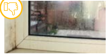
Uninsulated window with condensation.
