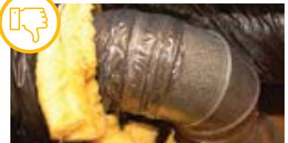
Flex duct is not mechanically fastened to metal duct.
