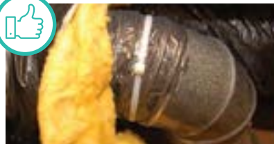
Flex duct is properly fastened to metal duct with mechanically tightened strap.
