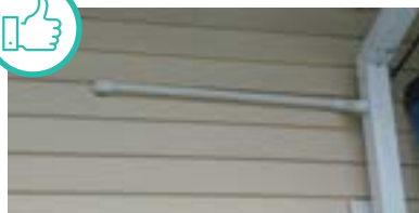
Condensate drain is connected to downspout.
