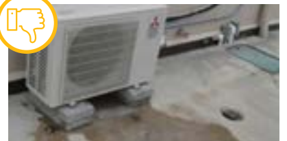
Condensate directly leaks onto a walkway.
